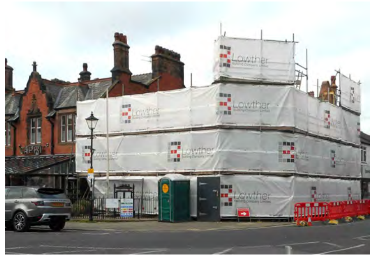
Was this the new Kentucky Fried Chicken outlet as rumoured around the town while the scaffolding was in place? (photo David Forshaw)
